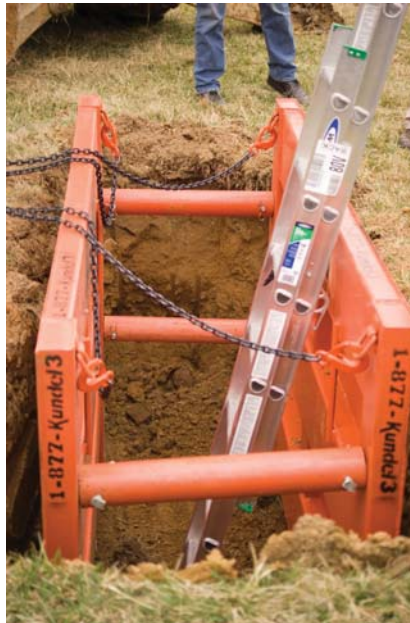
Do not enter a trench without inspecting it at the start of a shift or after a rain shower to ensure that all safety precautions are still in place.
