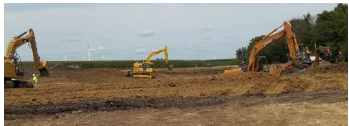
(above) Installation of control structure at the outlet for the Bureau County wetland. (below) 2 more action photos from the Bureau County wetland project last year, aerial shot of 2015 FPS tiling installation, courtesy of Chris Kaufman, SFDI.
