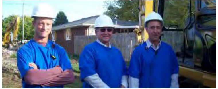
(Above) Carl Baer, Wayne and Jeff Litwiller, of Litwiller Excavating (Left) Dumping Gravel on top of fabric underlay for the new access road (Lower left) Beginning of demolition at the front of Gry's home. (Page 13, Upper right) Ty Pennington climbing into rubble for filming session. (Center) Excavator buckets making short work of debris. (Lower right) Start of basement excavation.
