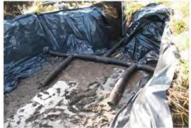
Manifold across width in lined bioreactor
